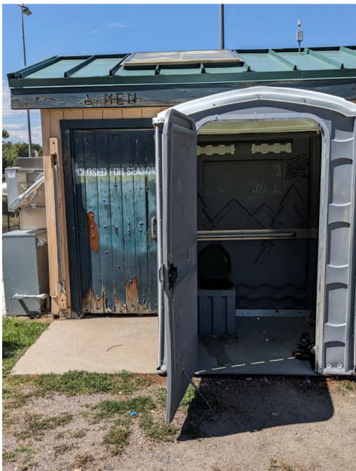
An example of a closed plumbed bathroom replaced by a porta potty at Rude Park. The photo was taken during the summer, even though the plumbed facility says that it is only closed seasonally.
